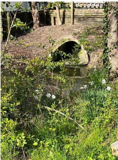
Storm drains from Route 1
