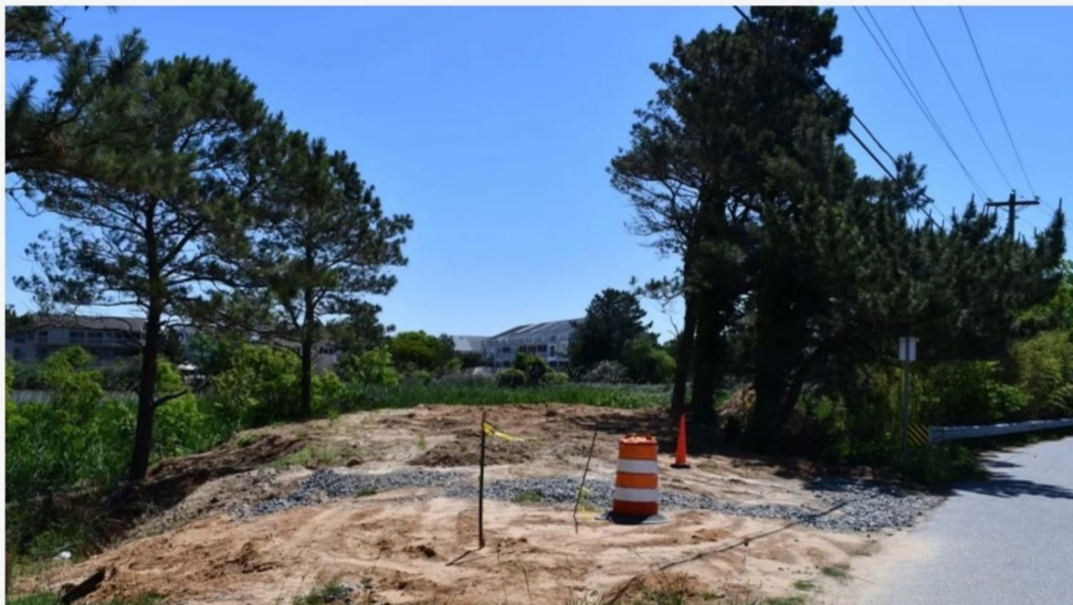
This land, on the southwest corner of Silver Lake in Rehoboth Beach, was clearcut and backfilled. (Photo: Shannon Marvel McNaught, Delaware News Journal)
