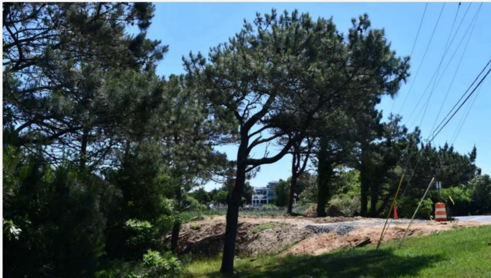
Dirt was used to raise the elevation of a property at the southwestern corner of Silver Lake in Rehoboth Beach, shown here May 30, 2024. (Photo: Shannon Marvel McNaught, Delaware News Journal)
